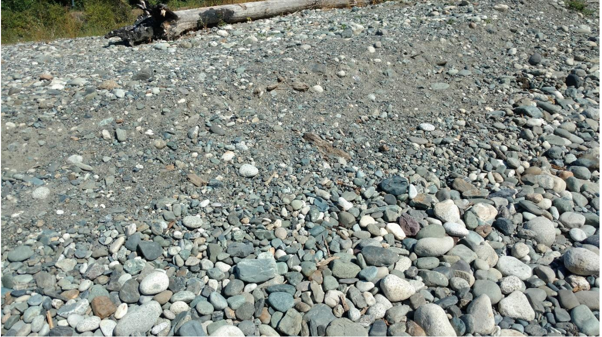
L2(a): LWD structure (LWD#L2016-2) placed along the bank-side of the pit upstream of LWD#L2016-1 in 2016 is gone. Picture taken on August 13, 2017.
