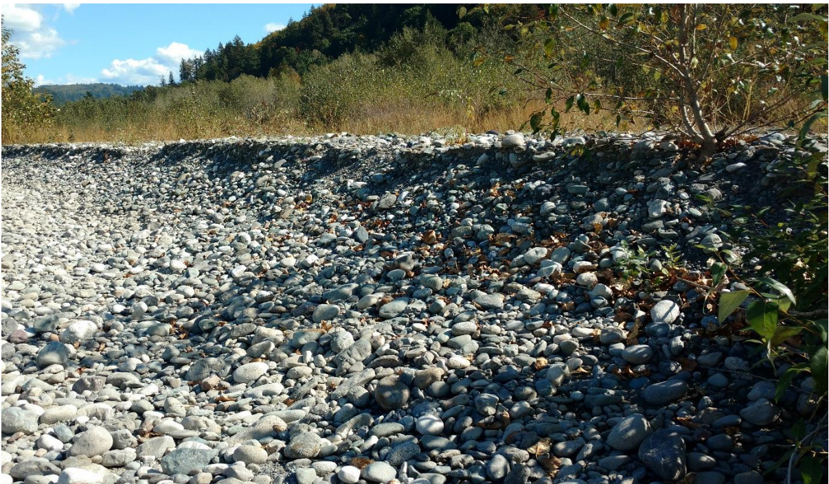
G3(a): LWD structure (LWD #G2016-3) placed in scalped pit along the bank-side is gone. A platform of boulders created downstream of LWD complex to enhance fish habitat is covered with gravel. Picture taken on August 13, 2017.
