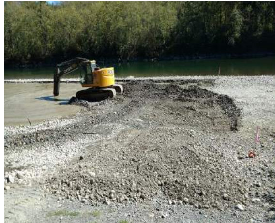
R6: Ongoing work activities, at downstream end. Excavation is near completion. September 12, 2016.
