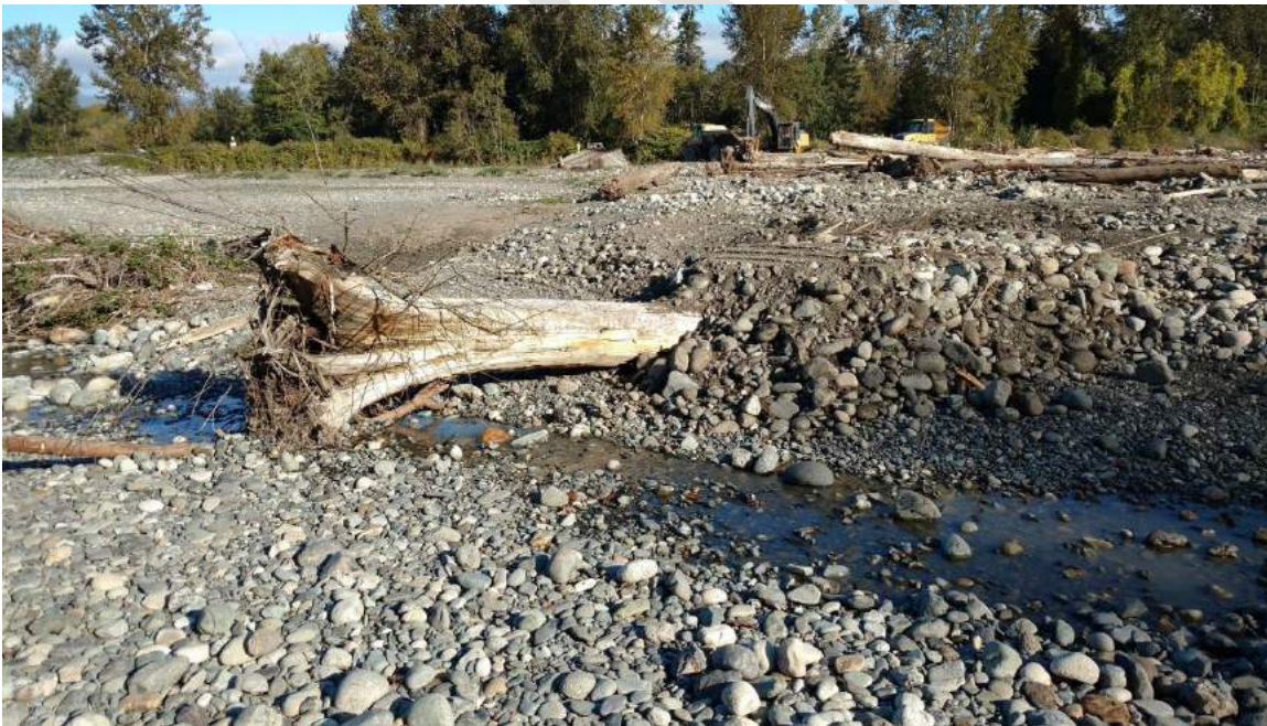
L4: LWD #L2016-4 –LWD structure placed in microchannel downstream of southwest outlet.
