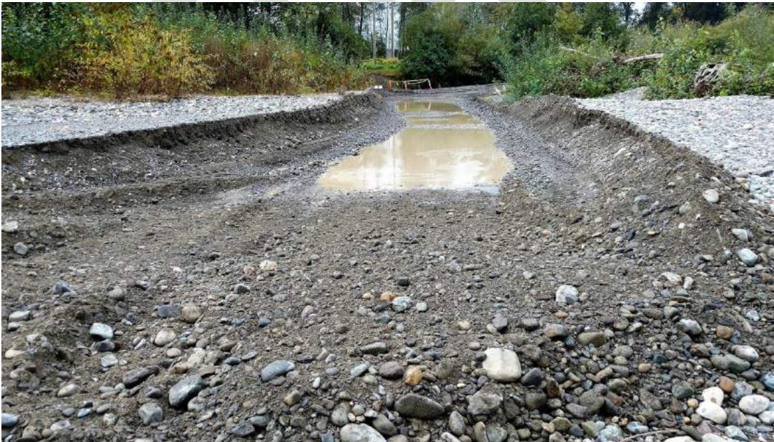
Upstream habitat excavation, work in progress. View towards left bank side channel. September 7, 2016.
