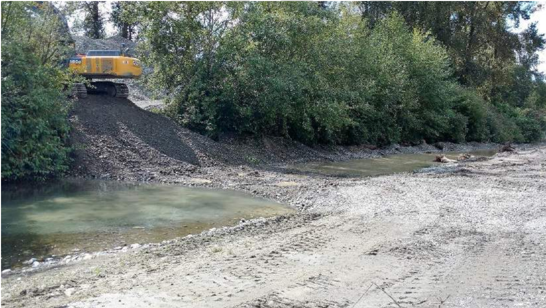
Left bank side channel reconnection with a 'riffle structure' after access ramp decommission. September 8, 2016.
