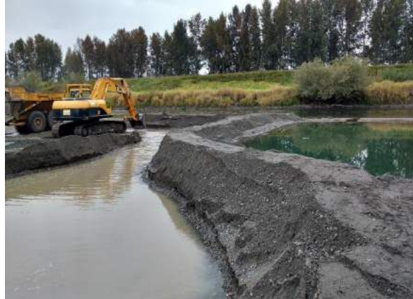
KW8: Berm constructed at upstream end and along the river to continue excavation after heavy rain. September 23, 2016.
