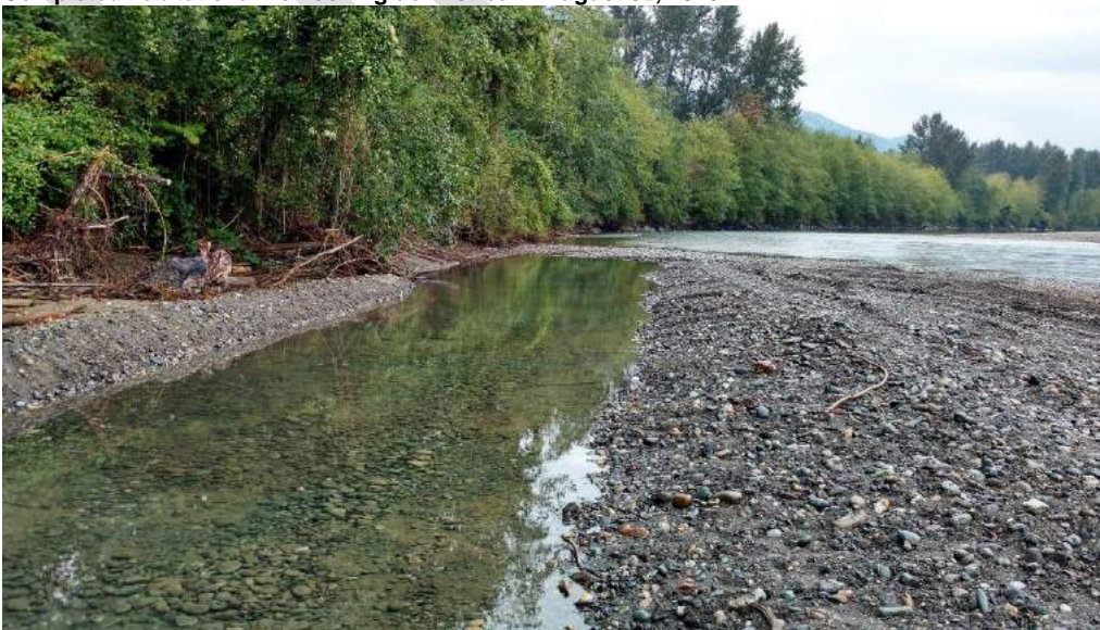
View of completed habitat channel at its downstream connection to the river. August 31, 2016.
