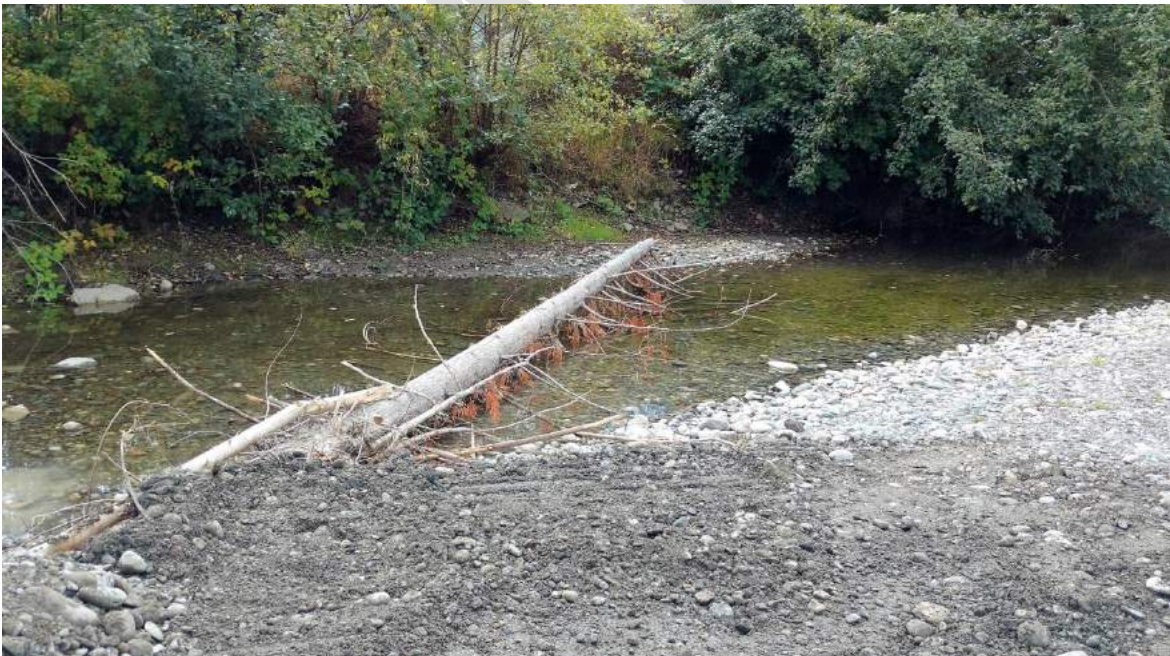
Y6: LWD #Y2016-6 –LWD structure placed along left bank side channel upstream of access ramp. Unlike more typical LWD placements, LWD #Y2016-6 and -7 were placed with the rootwad buried and the stem overhanging the channel. This avoided the need to disturb the flowing channel but still provided excellent cover.
