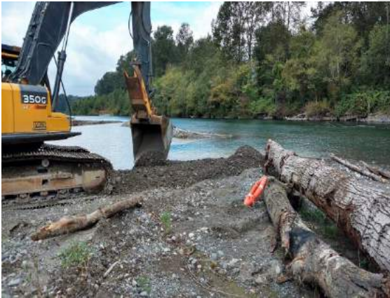
Y9: Constructing of inflow opening to the main river followed by outflow opening completion. September 8, 2016.
