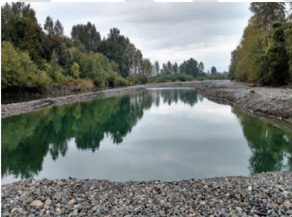
B11: View of the completed excavation from downstream of the work. August 31, 2016.
