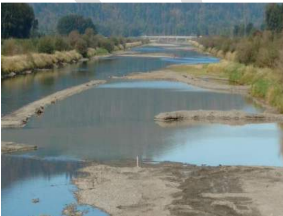
KW11: View of the completed excavation from upstream of the work. September 29, 2016.
