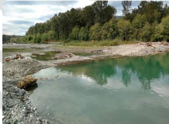
Y10: Third opening to the secondary channel at downstream end of the pit constructed as a riffle feature. September 10, 2016.
